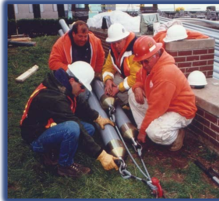
Tighten pulling eye so that it expands against the interior of the conduit.
