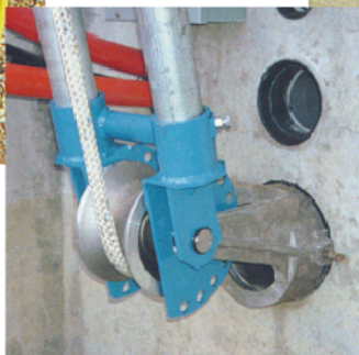
Duct End Joint
